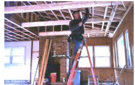
Carpenter John McCabe works on the ceiling of WPWA's conference facility, the final phase of our renovation project.
